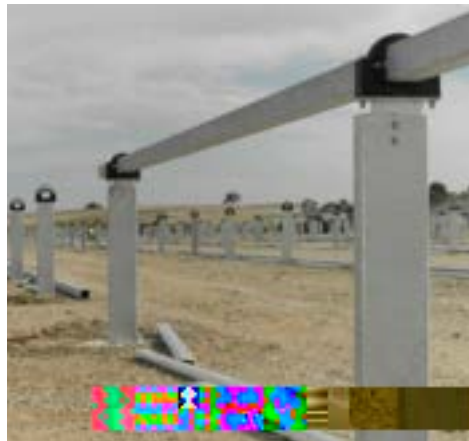
Spherical bearings installed in Zuera 11 MW, Zaragoza
